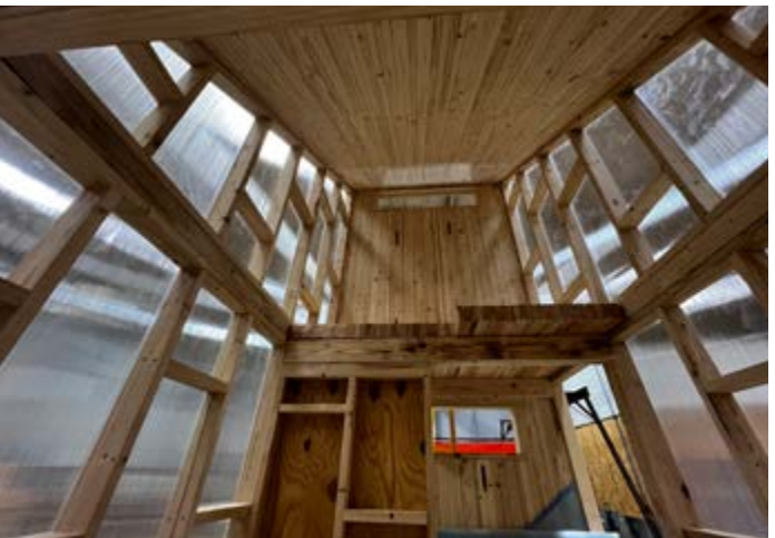
An interior view of the full-scale mockup with polycarbonate enclosure panels to be used where traditional framing is employed.
